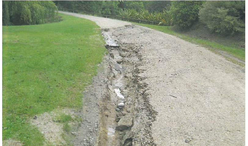
The damage caused by scouring from extreme weather events is clear in this example from 2013.
